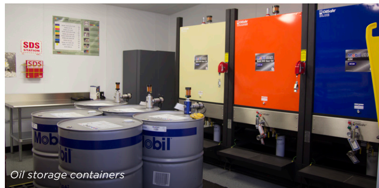
Top-up containers and grease gun storage
